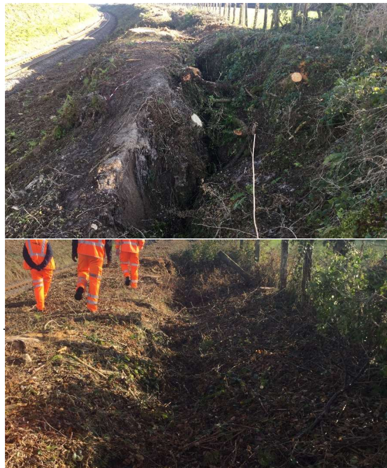
ABOVE: Views of the initial site conditions with no formal drainage systems, resulting in erosion of earthworks
