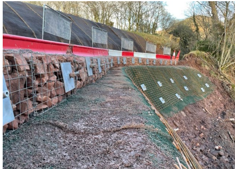
TOP: 13t excavator installing first row of nails for anchored gabion baskets by Griffiths roped access operatives.
