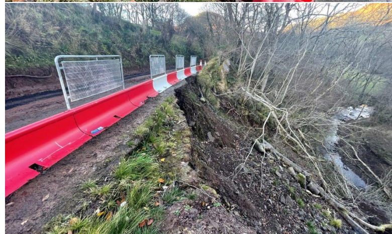
Pictured above: Views of the initial landslide from North and South perspectives, showing undercutting of carriageway.
